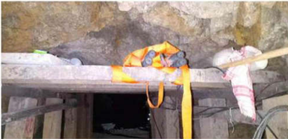
Fig -20. Stracher Provided for Drift Tunnel for Emergency
