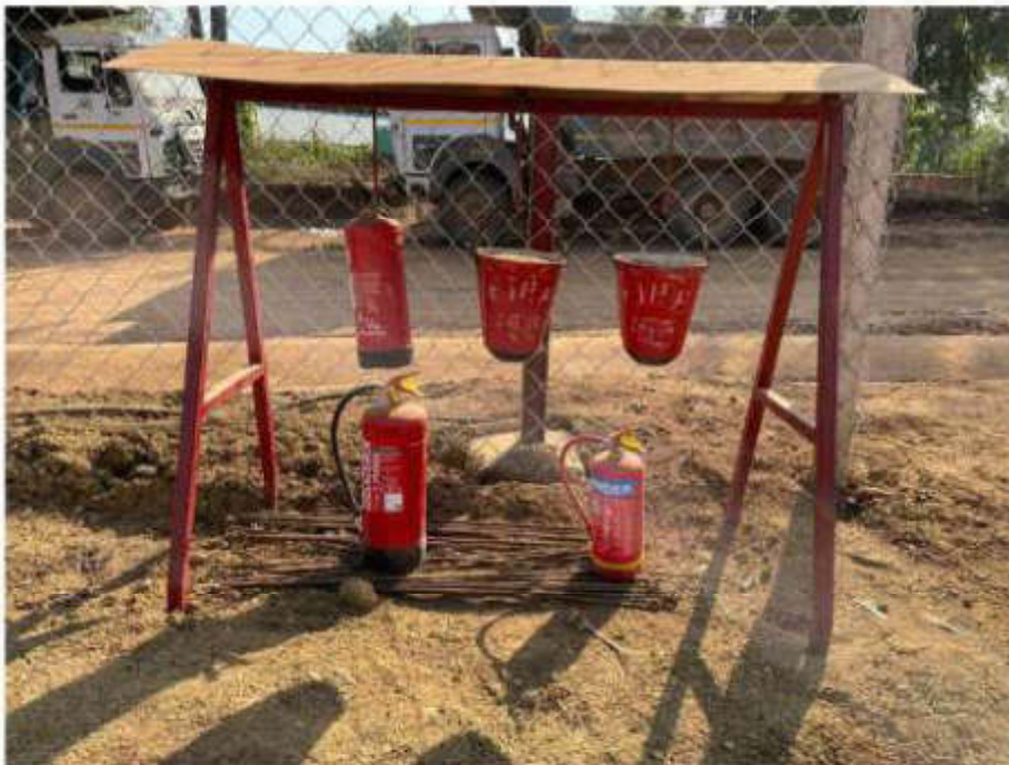
Fig -14. Fire Extinguisher provided for Fuel substation
