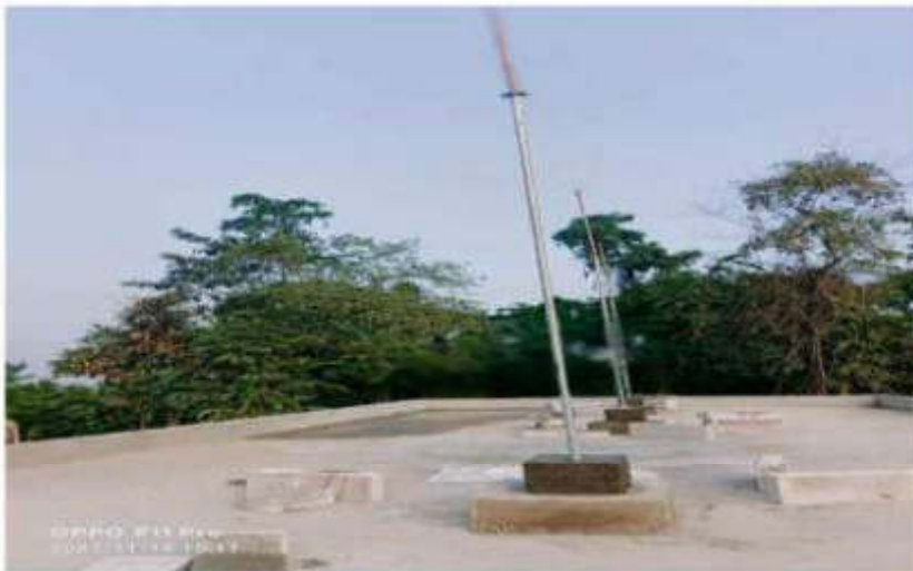
Fig -9. Lightning Arrester installed on Explosive Magazine
