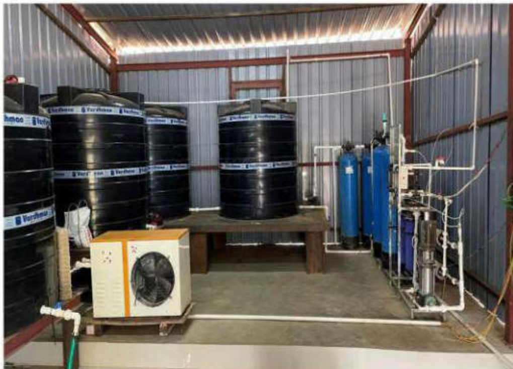
Fig: Installed 2,000 liter/hour capacity RO water plant for drinking water supply to all staff & workmen.
