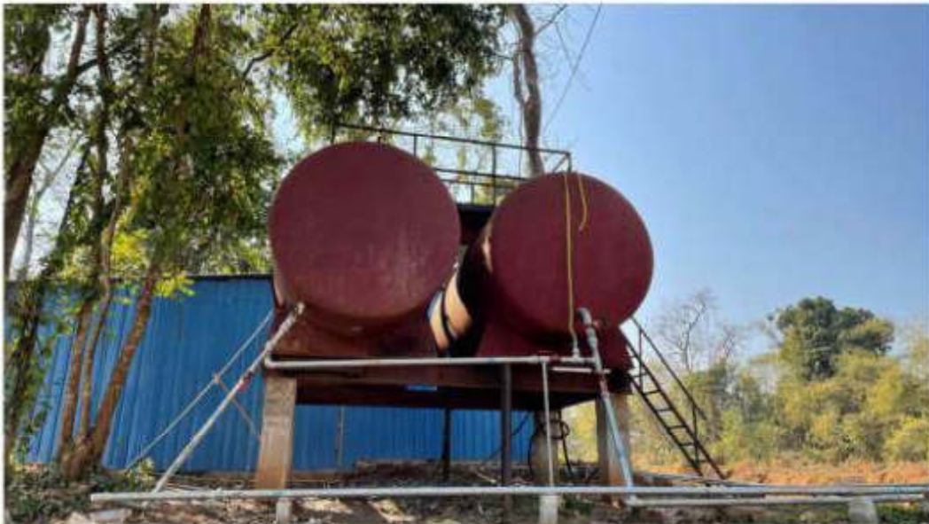
Fig: Water Storage tank one for treated water and second for waste water collection from RO plant, which will be use for non-drinking purpose (sprinkling, gardening & dish washing in mess)
